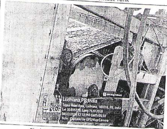
Sludge Thickening Process (Filter Press)
