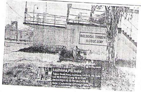
View of Biological Sump
